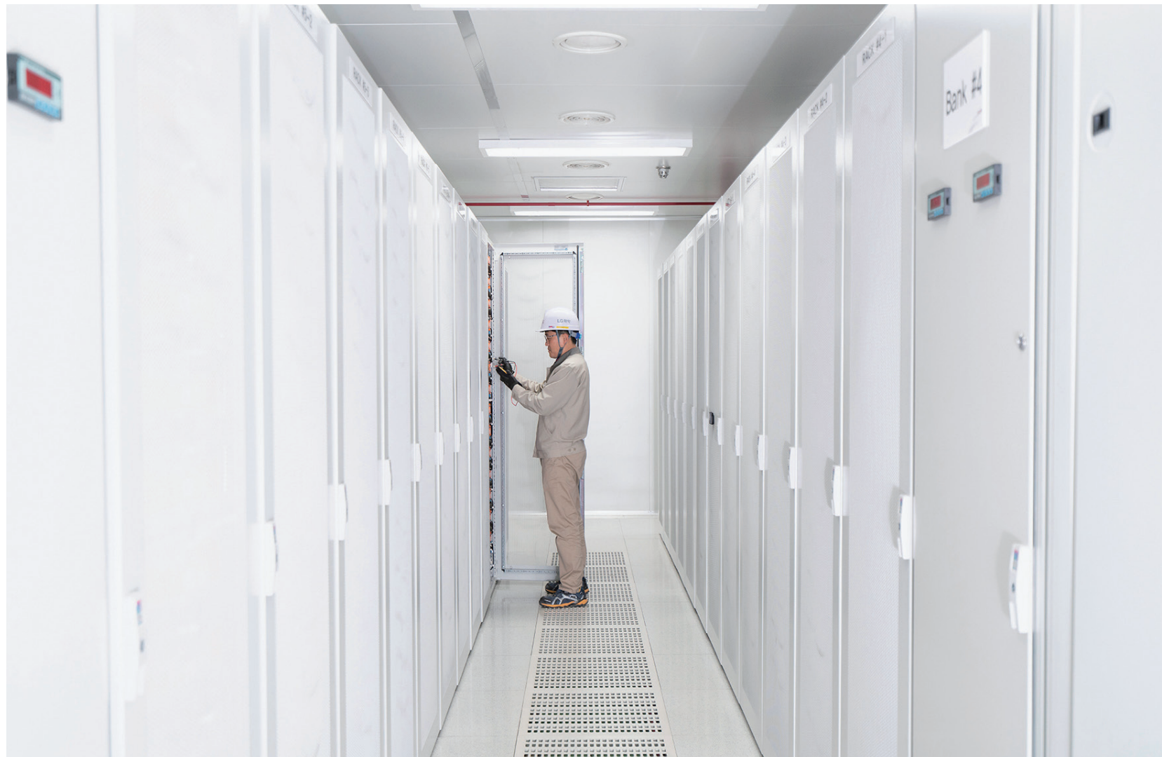
ESS operation management in Ochang Plant
