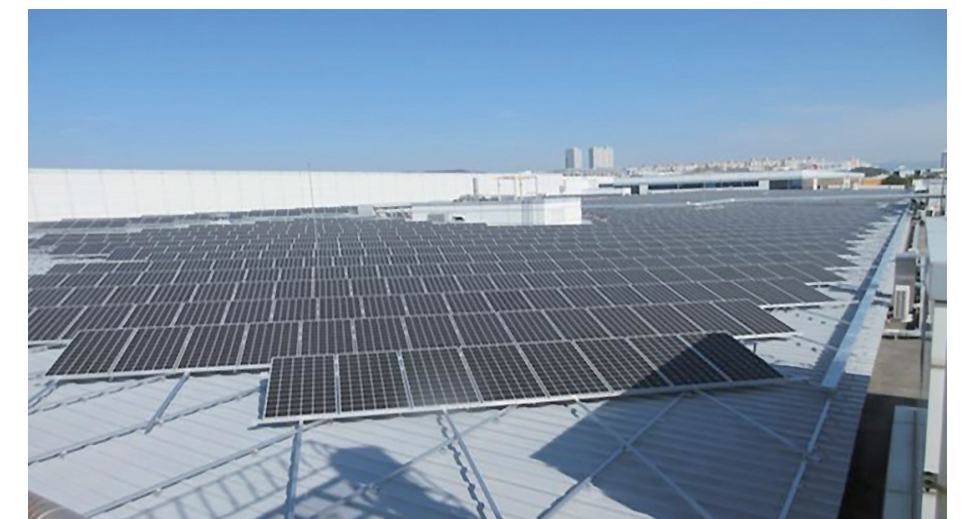
Photovoltaic system in Ochang Plant
